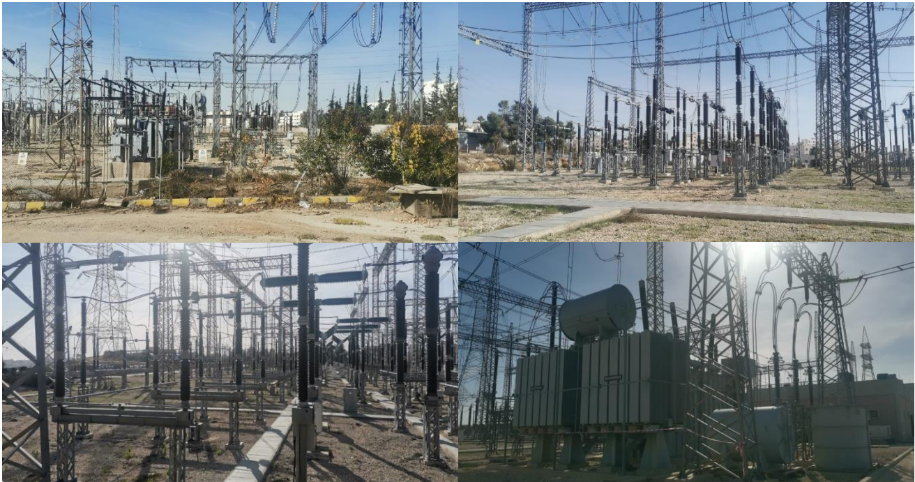
Figure 4: Typical View of a Substation
